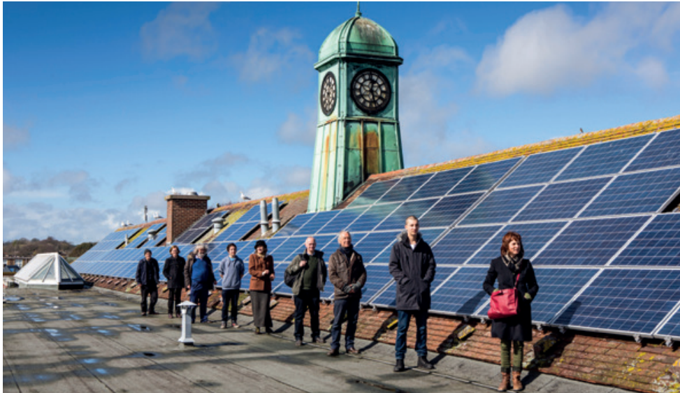
Ovesco investors on the roof of Priory School in Lewes, which will generate around 35,000Wh per year. It is one of five Ovesco sites.
